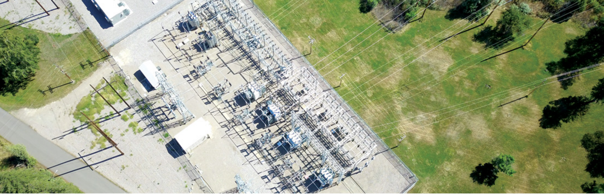
MVP power substation.
